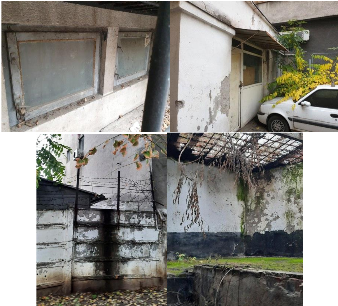
Fig. 5 - Lack of maintenance of outdoor spaces (facades and carpentry of main body C1, and the garage)
