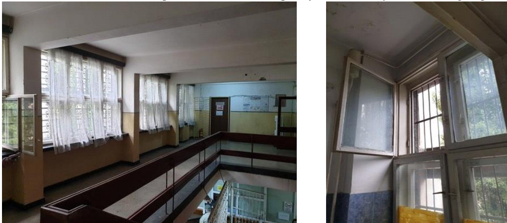
Fig. 6 - Lack of maintenance of outdoor spaces (yard walk, fencing)
